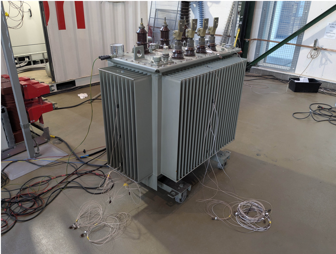
Figure H.6.: Full view of the transformer and placed sensors
