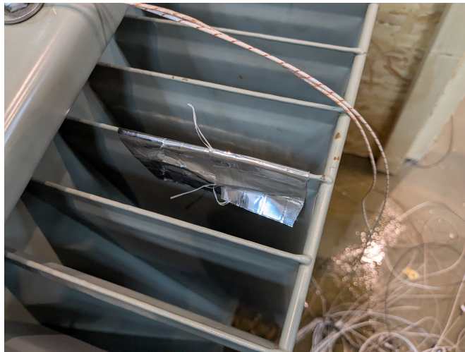
Figure 5.6.: Detached thermocouple Nr. 2 "Fin Top" on the short side of the transformer
