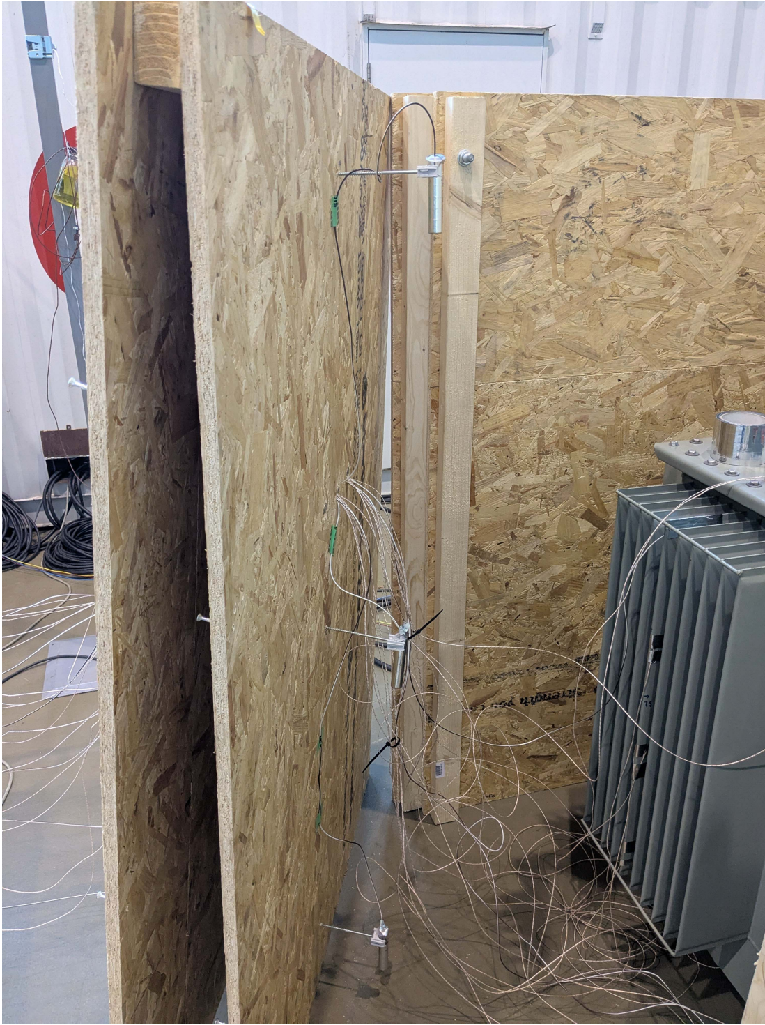
Figure H.12.: Sensor locations for air temperature inside the vault
