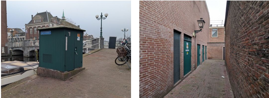
(a) Old type of compact substation, no longer placed. (b) Outside of indoor substation. Usually deployed when no space is available elsewhere.
