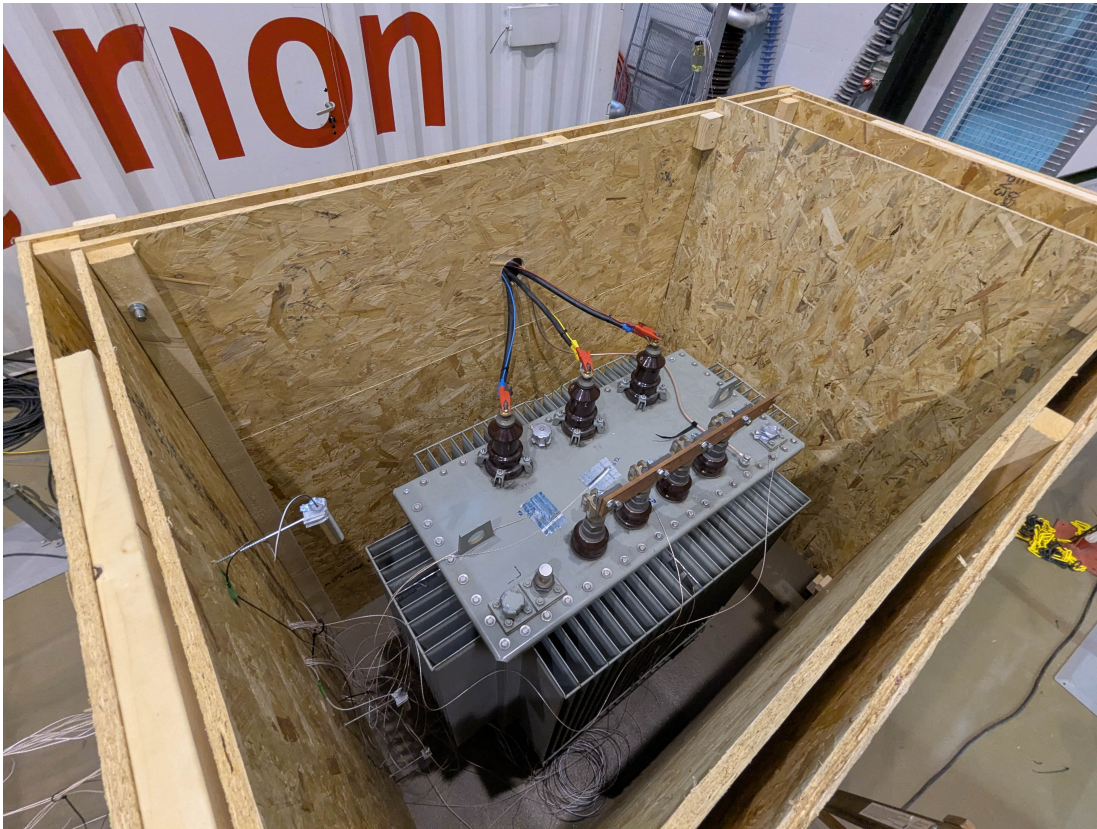
Figure H.2.: Transformer in Vault
